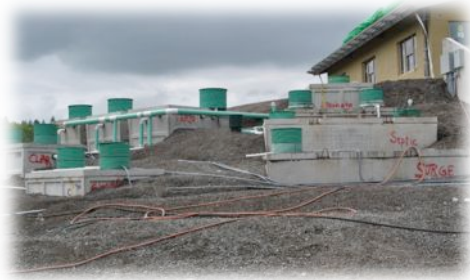
Gray water flows through biodigesting tanks before entering biofilters.
